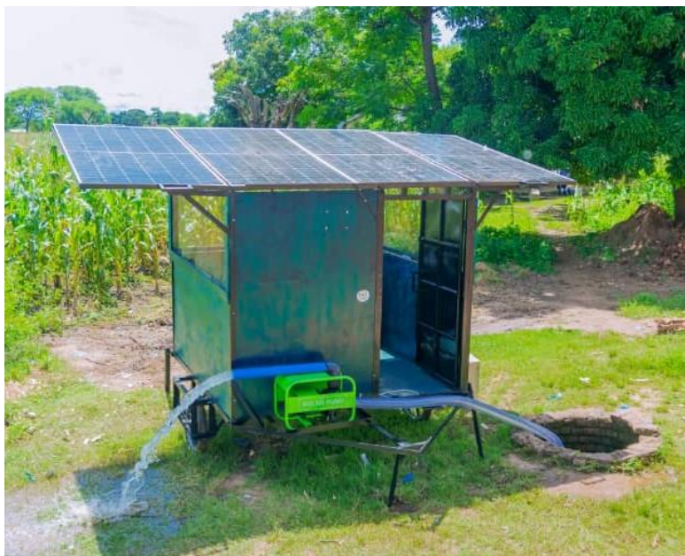
Figure 72 Kanyumba Solar Pump Irrigation system
